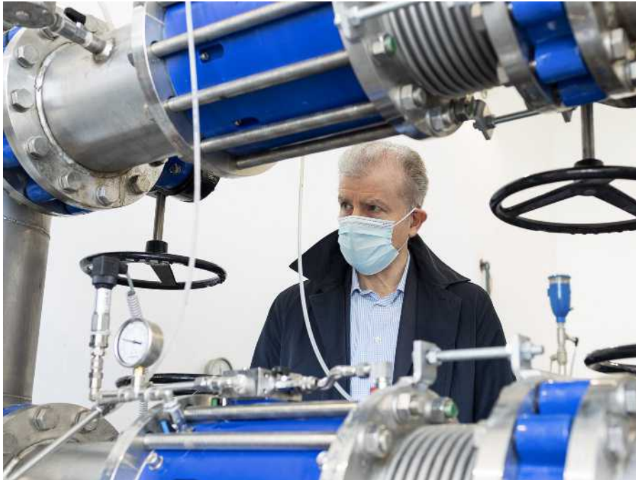
Marco Alberti, Sales Manager at GF Piping Systems Italy, checking twin pressure-regulating valves to control downstream pressure regulation.
