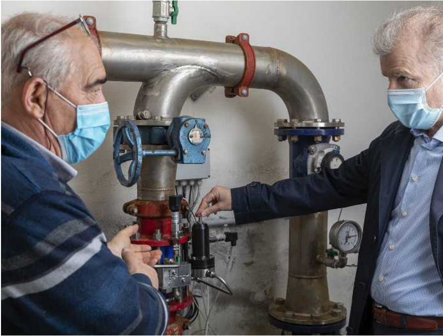
Antonio Gualtieri (L), Technical Manager for Water Leakage Detection at IRETI, and Marco Alberti fine-tuning the pressure regulating valve.
