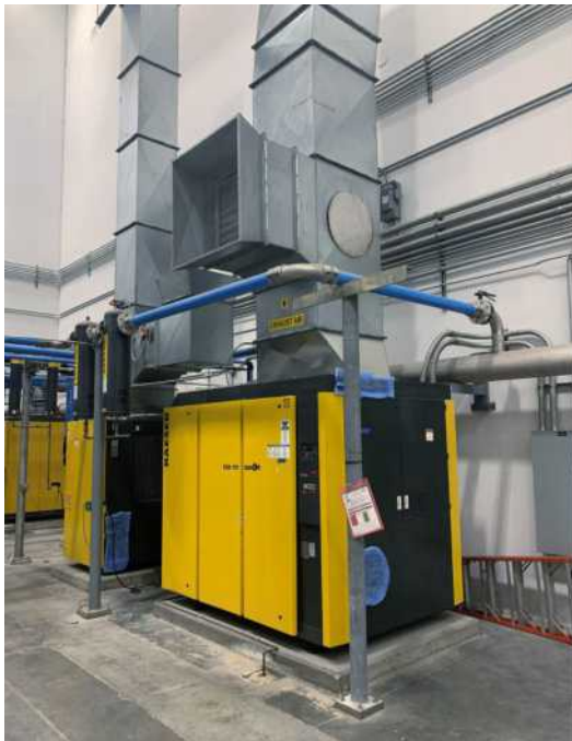
A new heat exhaust from air compressor at GF Linamar in Mills River.
